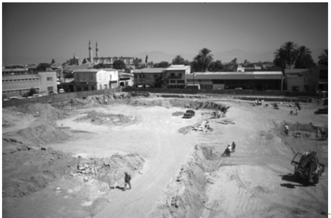
Early historical phases of Nicosia found at new Parliament building site, from the Late Chalcolithic period (mid-3 rd millennium BC) to the present day
